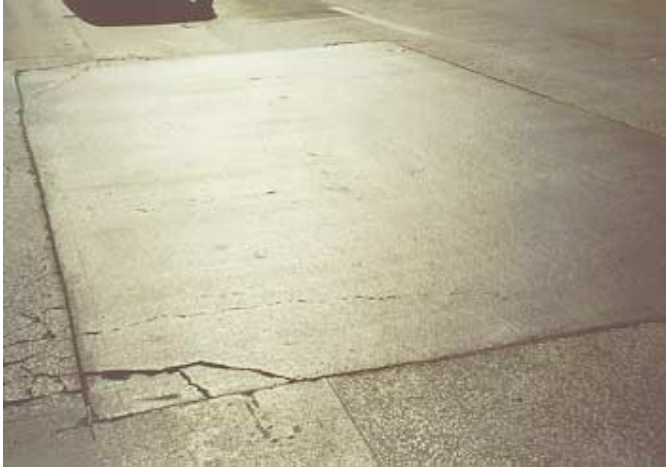
Fig. 3: The conductive-concrete patch after 12 months. There was no evidence of corrosion, but some reflective cracking
