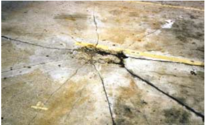
Fig. 1: Slab distress due to misplaced reinforcing bars
