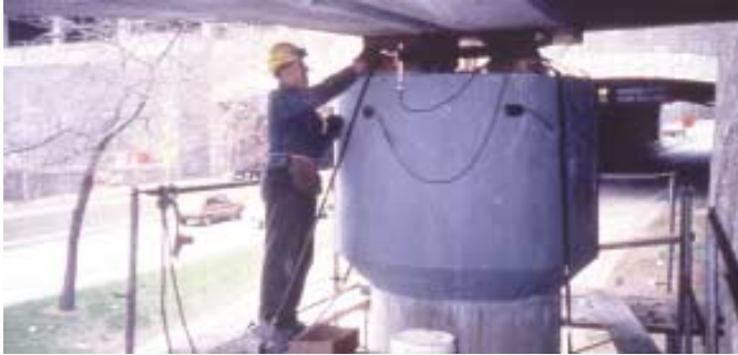
Fig. 12: Shear collar on top of a bridge pier provides a jacking surface for bearing replacement
