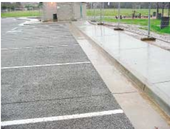
Fig. 1: A pervious concrete parking lot at Bannister Park, in Fair Oaks, Calif., allows rainwater to pass through the concrete surface. Note that joints match up with those in the sidewalk (photo courtesy of the California Cement Promotion Council)
