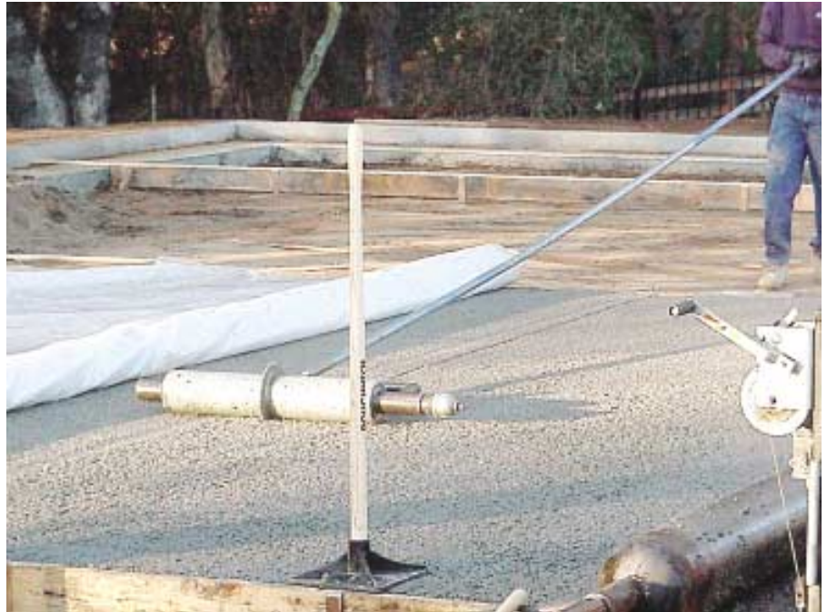
Fig. 2: The crew used a steel roller with a flange welded to it to create joints in the wet concrete. The roller-compacted surface required no further finishing, leaving a pebbled, open surface (photo courtesy of the California Cement Promotion Council)
