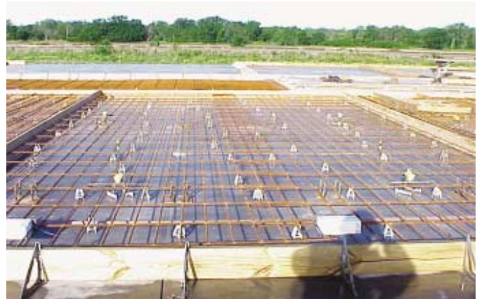
Fig. 3: Tilt-up panel reinforced with only WWR mats (Photo courtesy of CON/STEEL Tilt-Up Systems, Dayton, Ohio)
