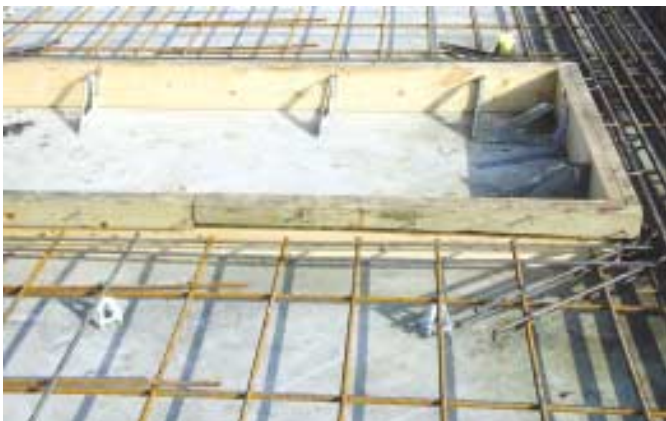
Fig. 5: Horizontal lap splice of WWR mats with loose vertical tie bar (Photo courtesy of CON/STEEL Tilt-Up Systems, Dayton, Ohio)
