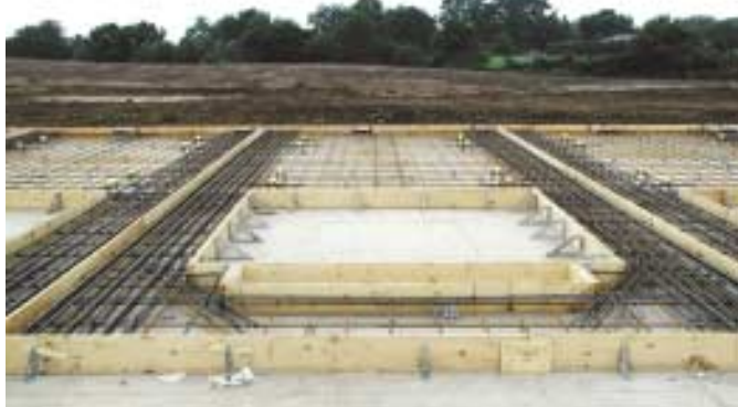
Fig. 2: Tilt-up panel with WWR augmented by conventional loose bars (Photo courtesy of CON/STEEL Tilt-Up Systems, Dayton, Ohio)
